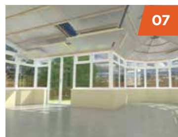
07 3 layers of high performance insulation (between and over rafters, and insulated plasterboard), is installed.
