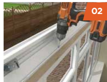
02 Timber packer and structural ring-beam are sealed and secured to the top of the window frames.
